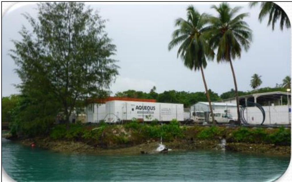
Figure 19: Example of Containerised desalination unit at a higher ground level
