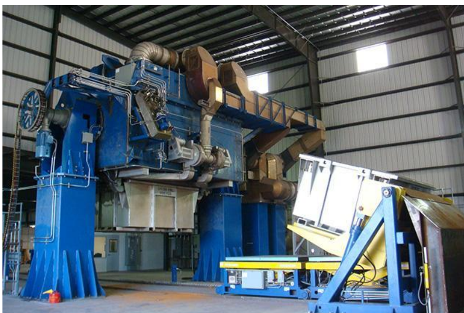
Interior Photo of the Chinook Gasification System
