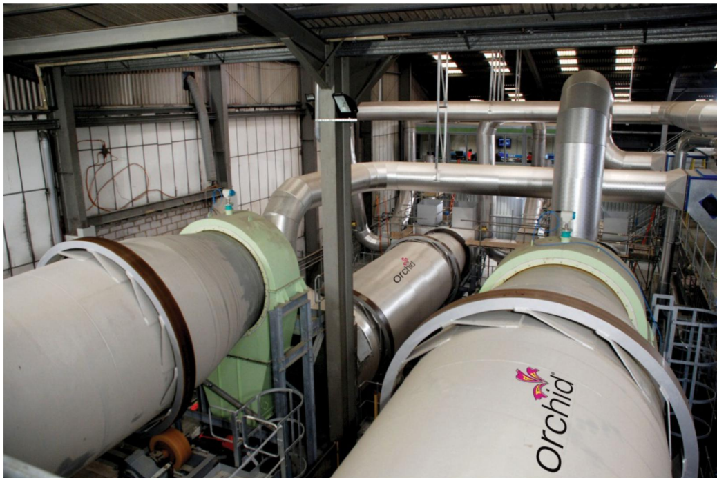
Interior of Orchid Environment Mechanical Heat Treatment Process
